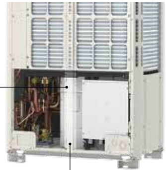
Compressor is enclosed in metal casing to reduce noise.
